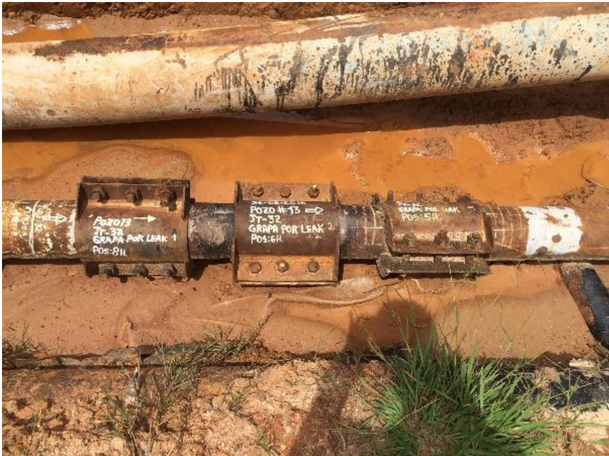
Photo 1: Pipe showing three clamps added following three pipe ruptures that led to spills.
