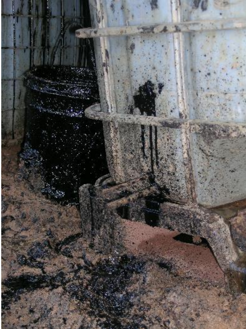
Photo 5: Storage tanks for oil spills that have broken; fissures allow leaks towards the Manchari River
